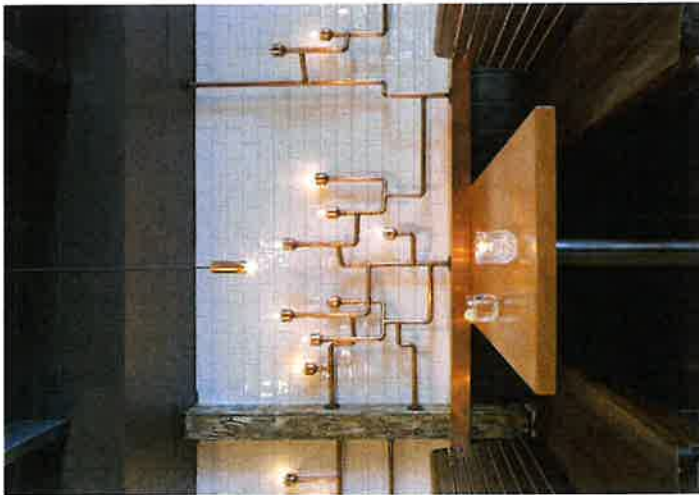
Copper pipe lighting for on the left wall on entry
